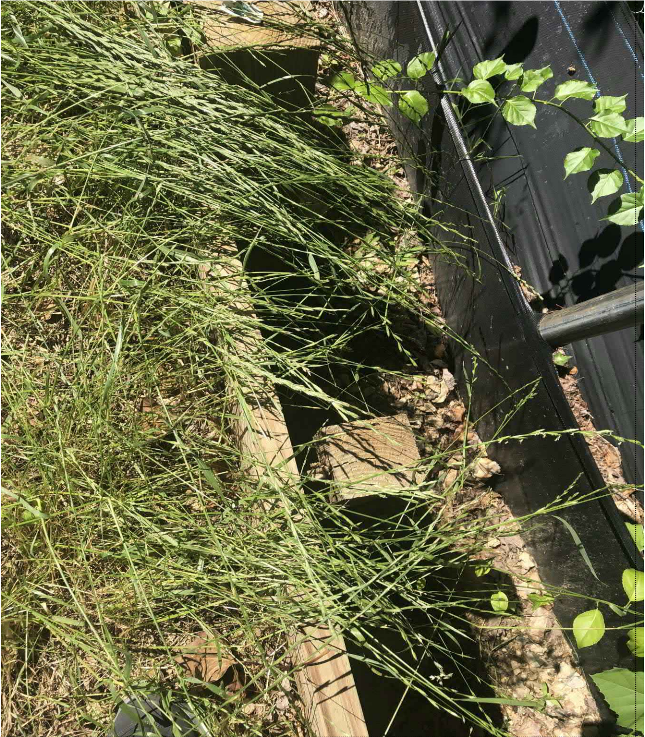
Sediment between Wall and Silt fence
