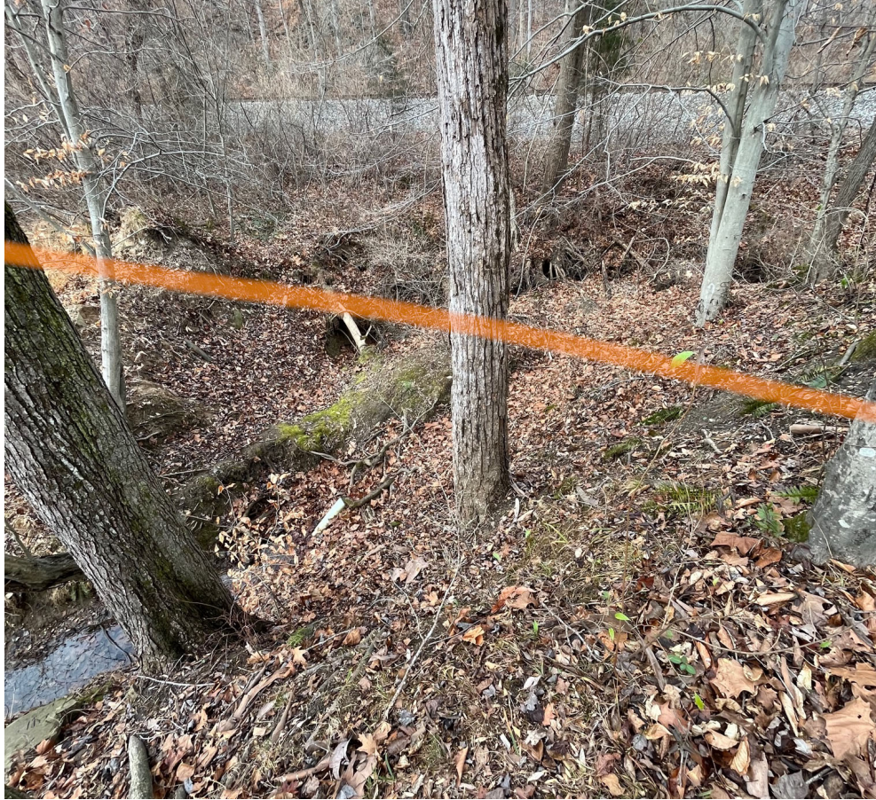
Damaged Embankment with proposed trail route (orange) 15
